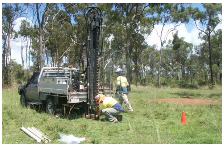
Geotechnical drilling that will be used to investigate ground conditions for the design
